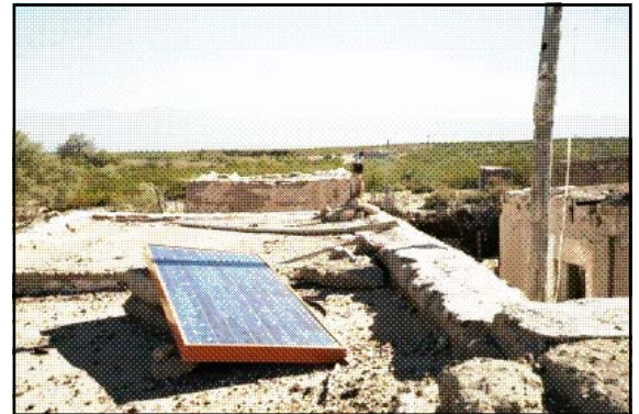
A rooftop solar panel captures renewable, clean energy.
